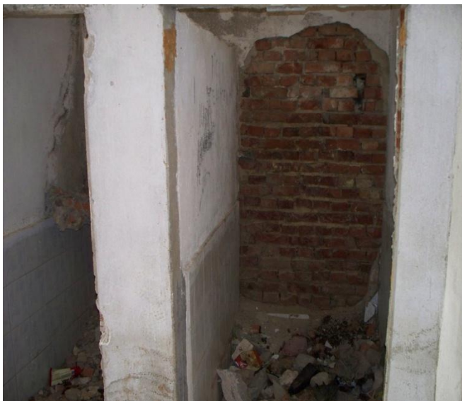
Figure 6: First floor restroom in its current condition.
