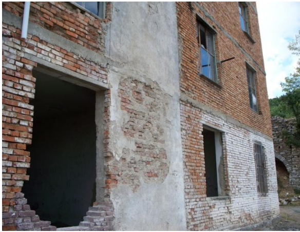
Figure 10: Alternate view of exterior with missing walls and windows.
