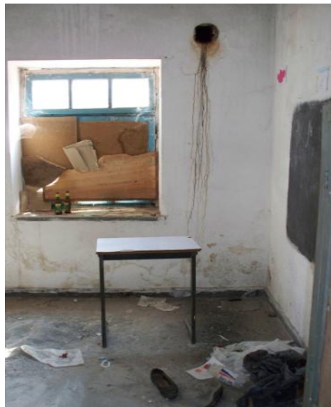
Figure 7: Detail of an unused classroom.
