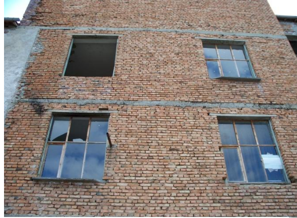
Figure 9: Alternate view of school exterior including windows in disrepair.
