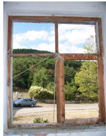
Figure 5: Example of a window in need of replacement.
