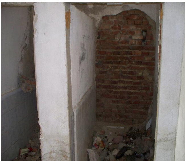
Figure 6: First floor restroom in its current condition.
