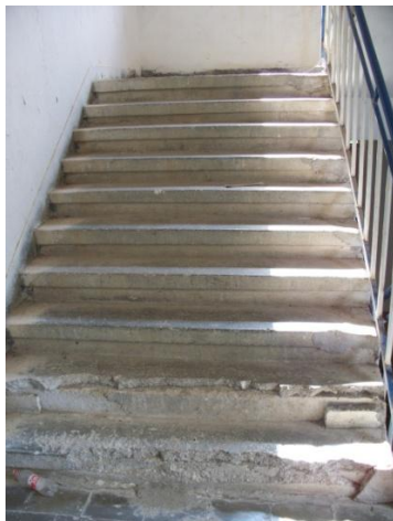
Figure 4: A main staircase in need of structural repairs.
