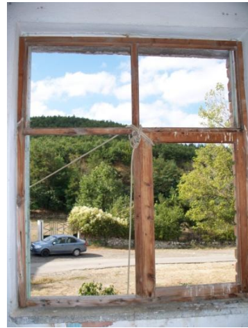
Figure 5: Example of a window in need of replacement.
