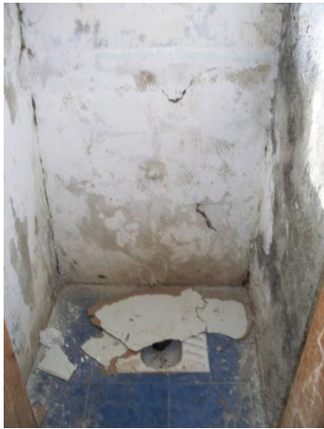
Figure 3: A restroom in its current state of disrepair.
